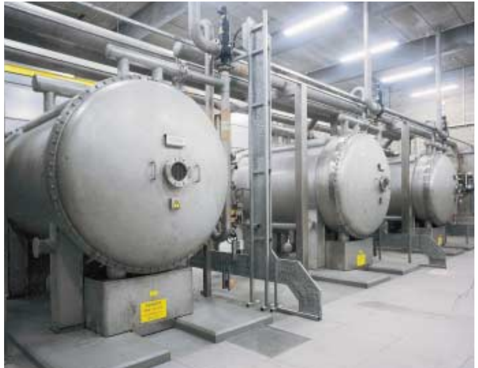
Figure 1: Coppermills Advanced Water Treatment Works Advanced ozone generators with a unit capacity of 48 kg/h at 10 wt%
