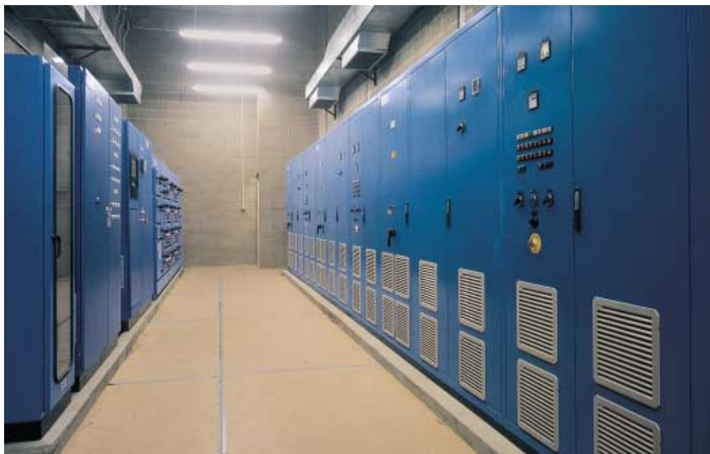
Figure 12: The control room of the Coppermills Advanced Water Treatment Works (GB) with the medium frequency power supply unit on the right
