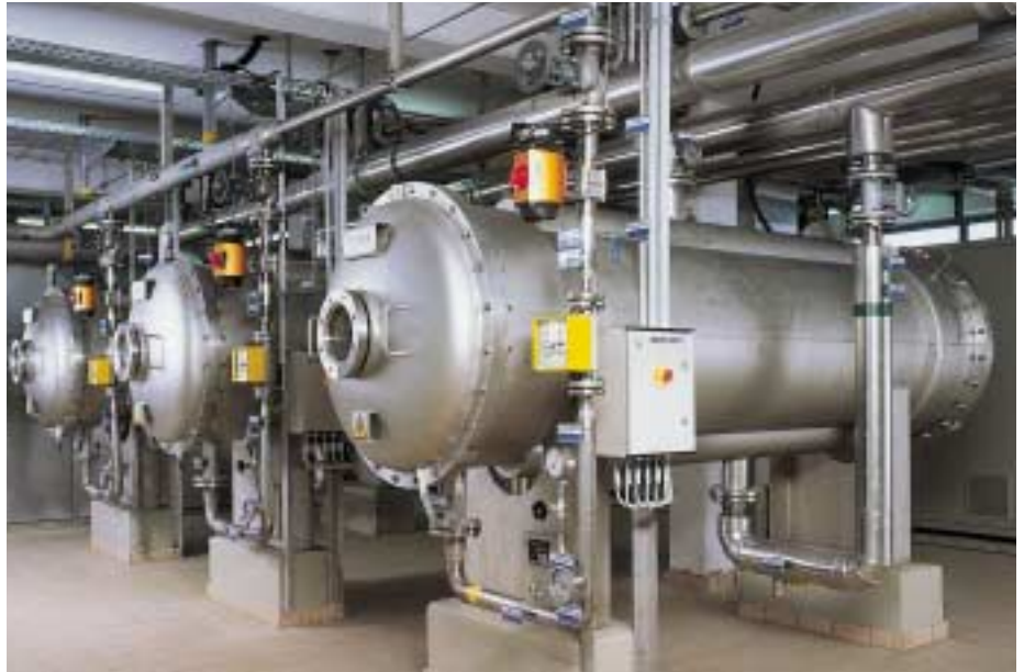
Figure 8: Rostock Water Works. Advanced Technology ozone generators (3 x 8.7 kg/h at 10 wt%)
